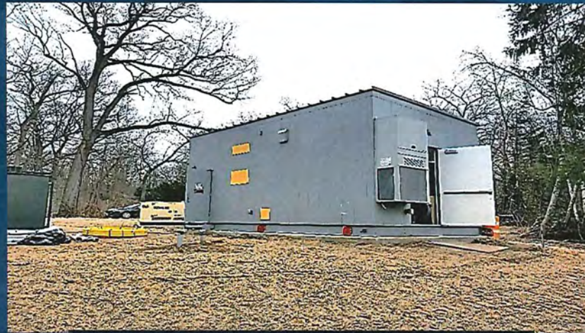
Replace Electrical Substation No. 45 ($1.6 Million)
